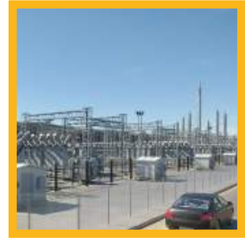
DEDICATED GRID STATION
